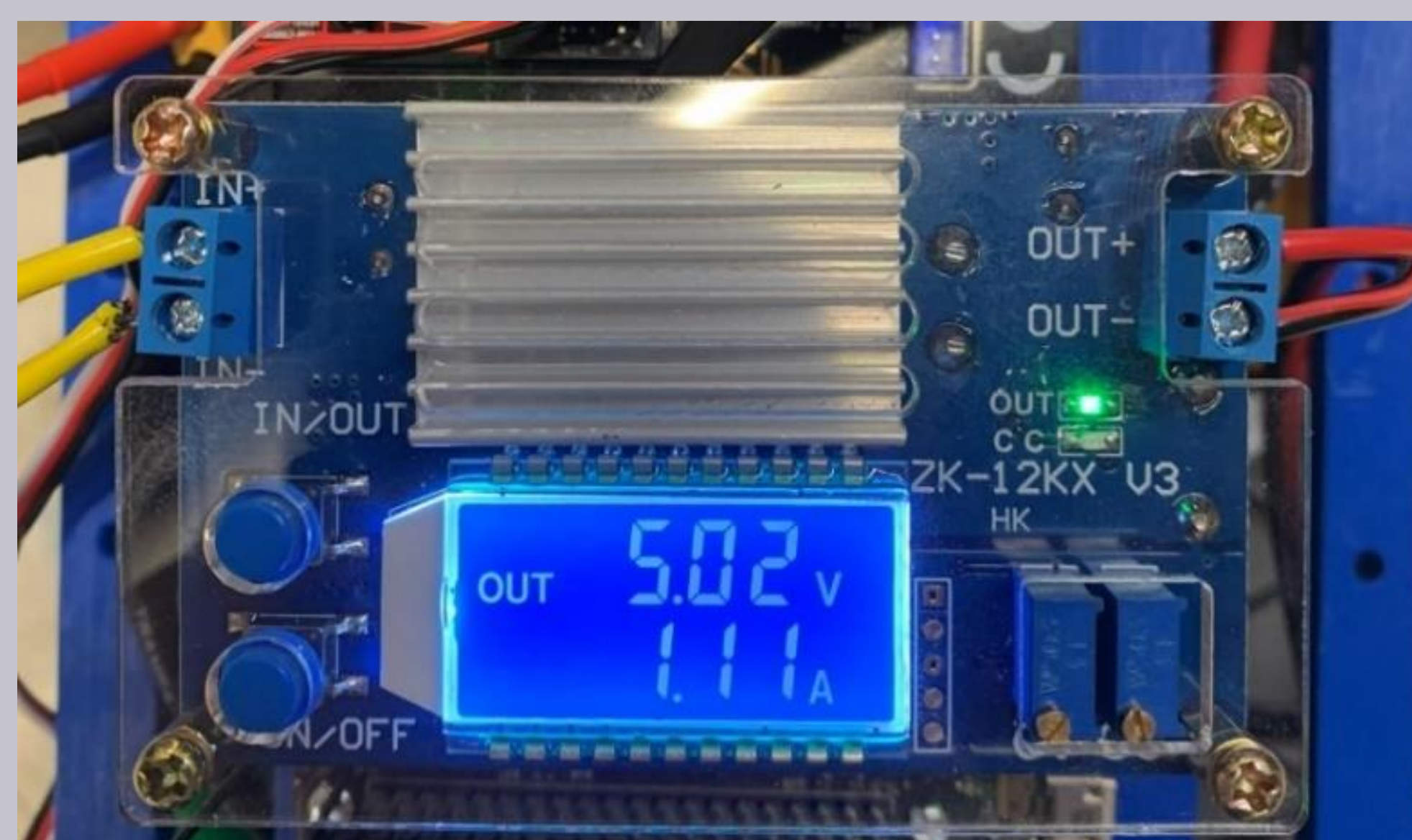
Figure 3: The power board's actual output current. Given the device's connected to the Jetson, we were expecting it to draw roughly 4A. The output current was much less than we anticipated drawing average 1.25A DC.
