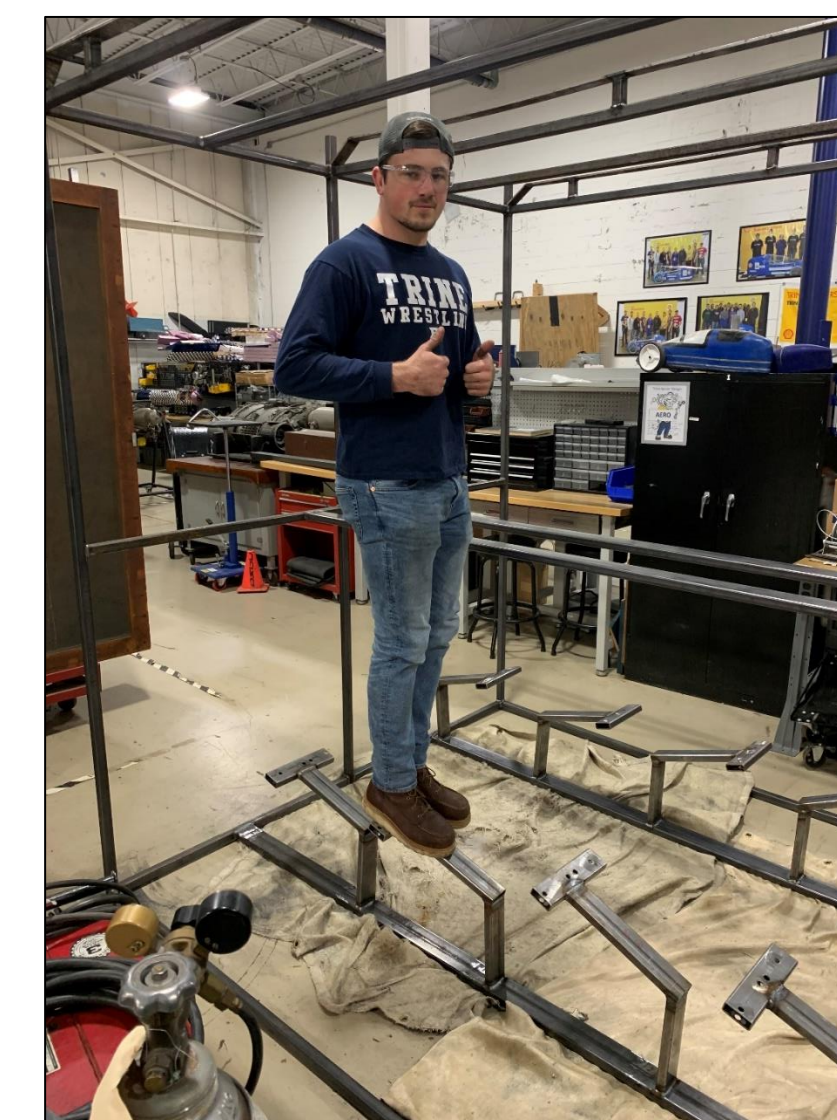
Figure 9: Shipping Crate Final Assembly Test
